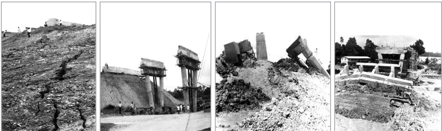
Cracklines in embankment.
