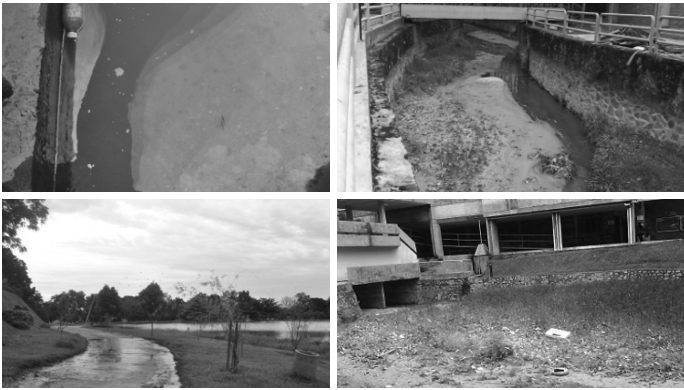
Figure 3: Erosion and sediment issues at Alur Ilmu UKM
