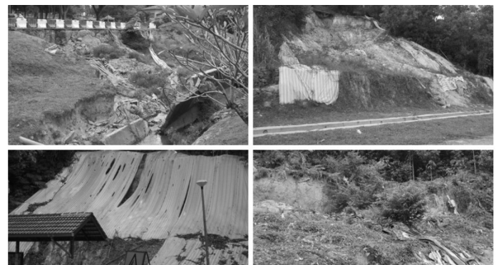
Figure 2: Landslides occurred in UKM Bangi Campus
