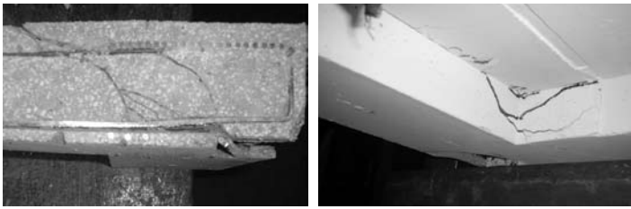
(a) Inclusion of internal cracks (b) Loss of failure surface
