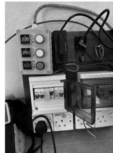
(a) Field test set with functional and faulty RCDs for simulation of fault condition
