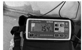
(d) Earth loop impedance test - Earthing rods with connection to foundation earth
