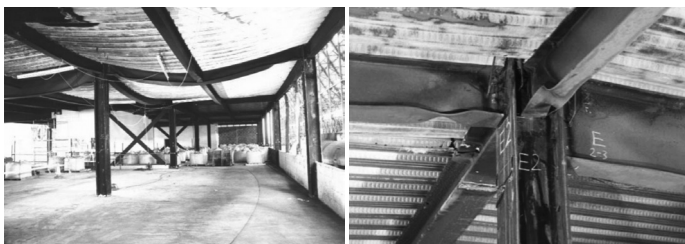
Figure 8: Ductile failure of steel structure due to fire (Bailey et al. [12], 1999; Allam, Burgess and Plank, 1999 [13]).
